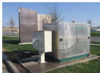
CrossIron Mills Shopping Centre
